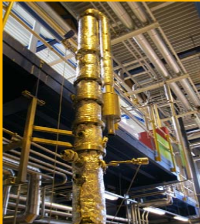
Stripper at the pilot plant
